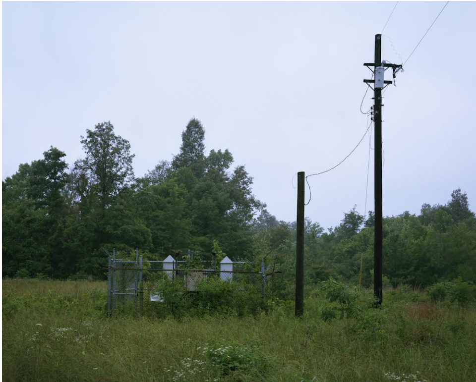
(Slide 3) Air Monitoring Station, WMA, Kentucky
